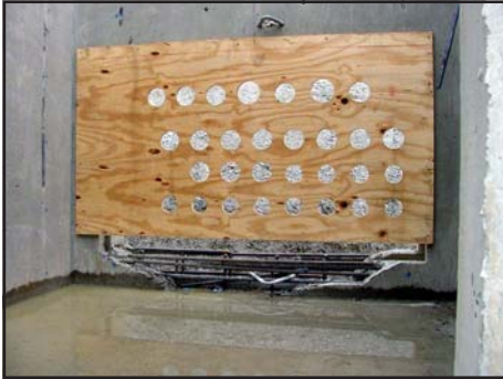
Poor flowability and rebar congestion led to exposed steel bars in the lower end of this manhole wall. SCC could have flowed easily to the bottom of the forms to prevent this situation.
