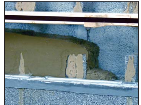
This close-up of the panel in the previous photo shows the leading front of the grout as it travels over a projection into the core, flowing around obstructions to fill the cells completely.
