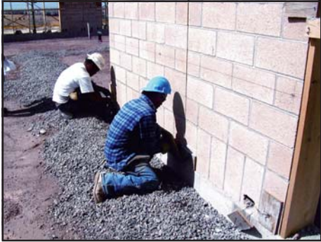
Cleanouts are used to assure that grout spaces are clean and free of debris prior to grouting.
