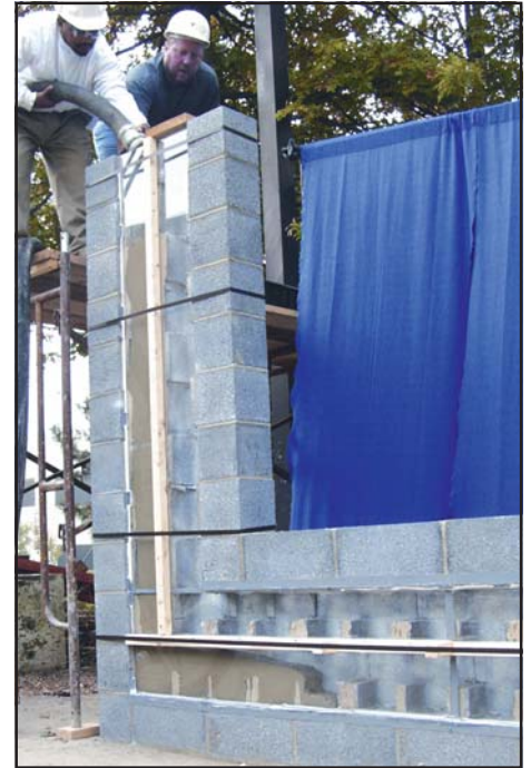
As seen through the clear plastic face on this demonstration panel, self-consolidating grout moves freely in tight spaces.
