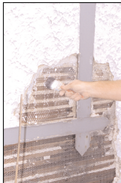
Figure 6. Applying a bonding agent can improve adhesion to the substrate and existing plaster. (69908)
