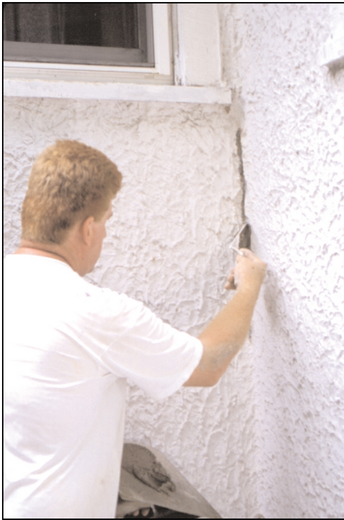
Fig. 8. Static cracks can be filled with a rigid material, such as a plaster finish coat or elastomeric coating. (69909)
