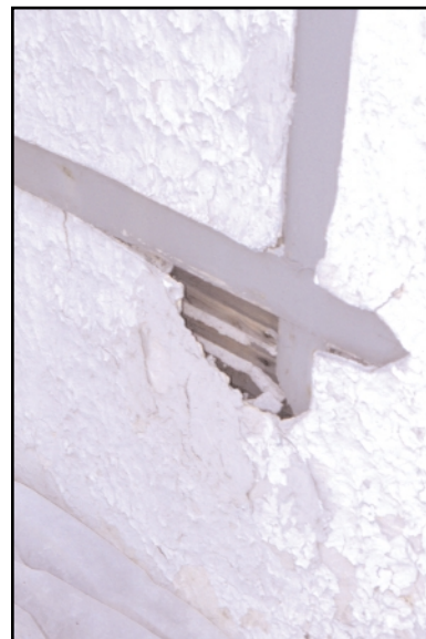
Fig. 3. Water-damaged plaster often bulges or falls away from the building. (69906)
