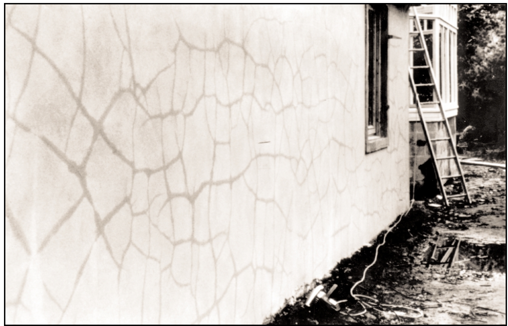
Fig 2. Improper curing of plaster can result in map cracking. (69914)
