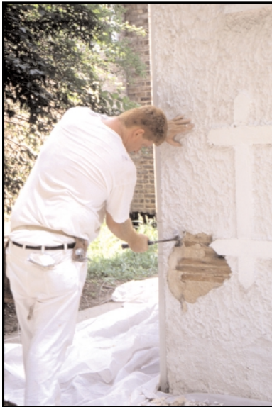
Fig. 4. Soft or crumbled plaster can usually be removed with a chisel or other hand tool. (69907)
