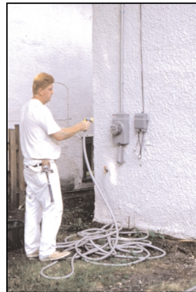
Fig. 9. Directing a high-pressure stream of water from a garden hose may be all that is needed to clean plaster. (69910)
