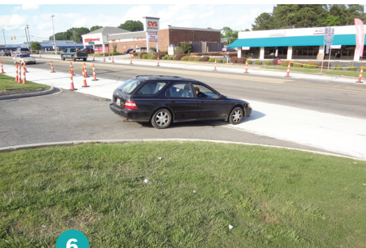
6 During the curing period, mainline traffic is kept off the RCC pavement, but crossing traffic is allowed at driveways
