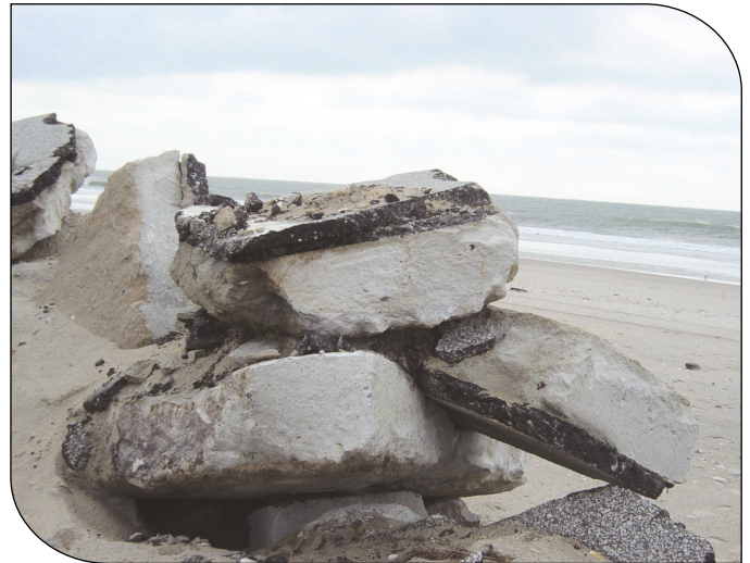
Hurricane Isabel undercut and fractured the pavement structure, but the soil-cement remained largely intact and bonded to the asphalt.
