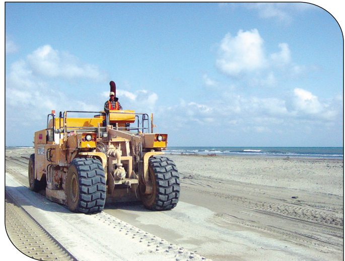
In some locations the old soil-cement base was still in place, and had to be reclaimed with 800-hp machinery.
