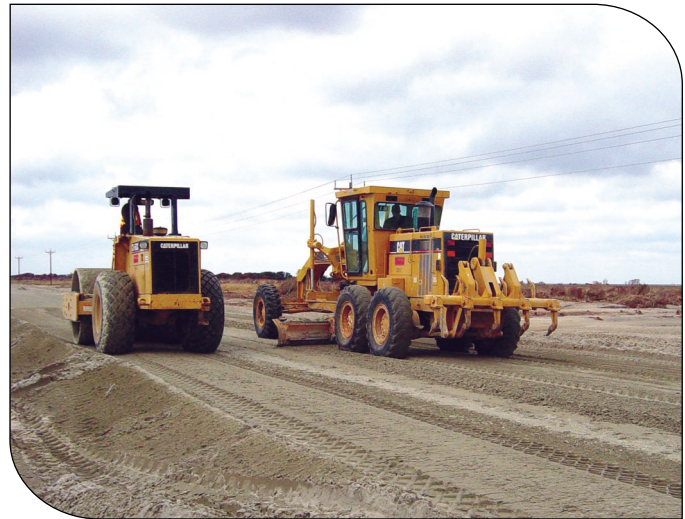
To avoid hauling aggregate materials to the island, crews compacted a mixture of beach sand and portland cement to form a sturdy roadbed.
