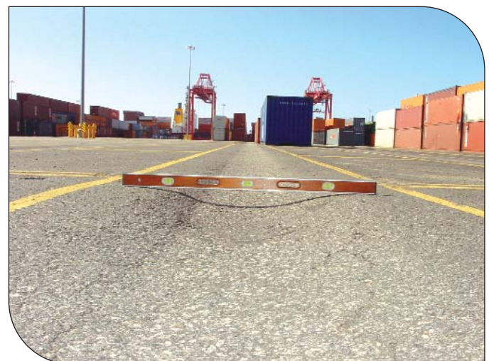
Rutting in asphalt pavement caused by channelized loading.
