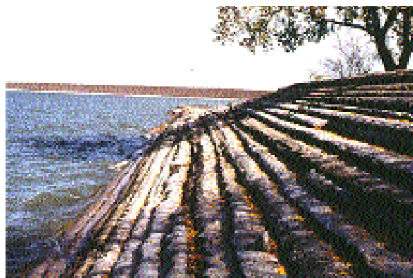
Figure 3. Condition of Bonny Reservoir soil-cement test section, 49 years after completion. (S#70033)
