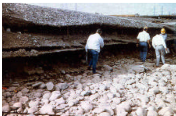
Figure 8. Erosion of cement-stabilized alluvium (CSA) bank protection on south side of Salt River at Tempe, Arizona following 1993 flood.
