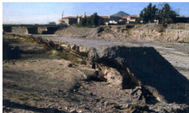
Figure 4. Soil-cement bank protection after overtopping during 1983 Tucson flood. (S#70037)
