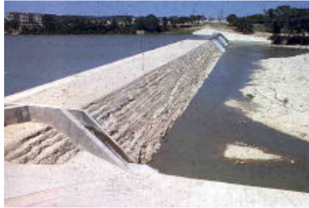
Figure 7. Condition of Kerrville RCC Ponding Dam after 1985 overtopping. (S#56065)
