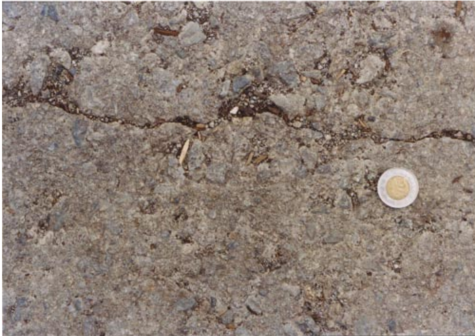
Figure 34 Typical RCC crack showing little deterioration. Joint sealer would be difficult to apply.
