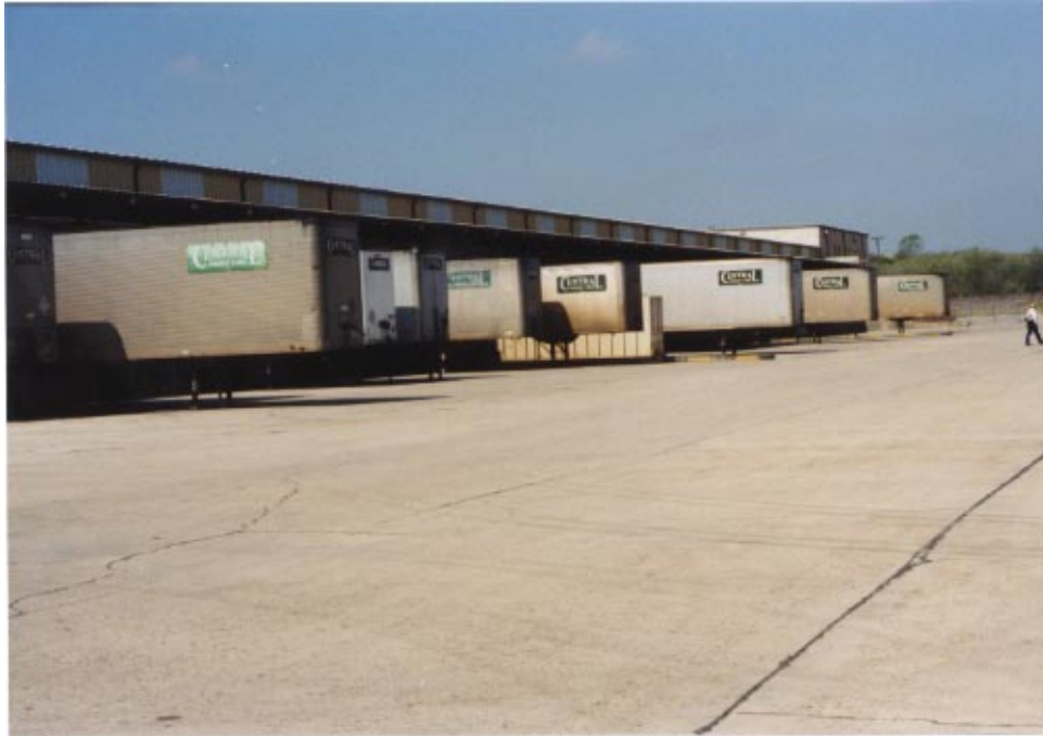
Figure 19 RCC truck terminal pavement at Austin, TX is in excellent condition after eleven years of service.
