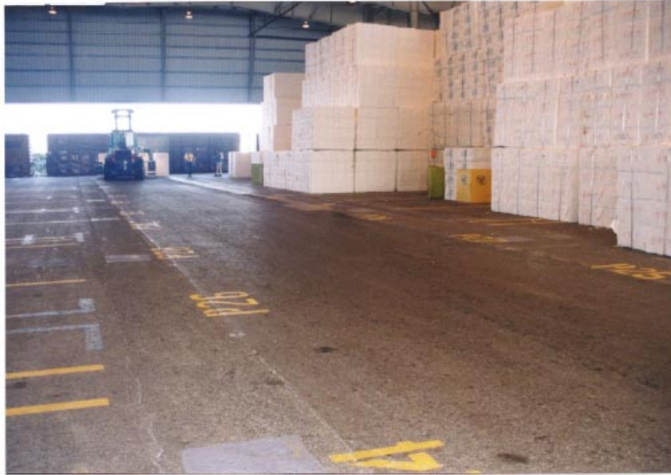
Figure 21 The RCC operating surface inside the warehouse where baled pulp bundles are stored.
