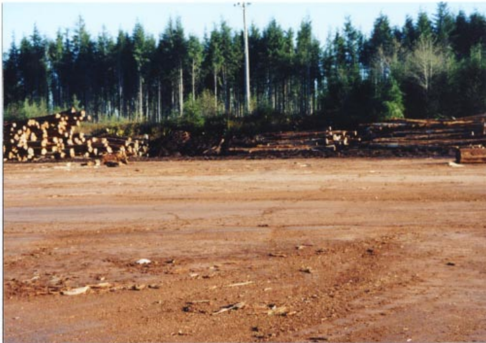
Figure 24 Though cracking of the surface is extensive, the log sorting yard continues in full operation after 20 years.
