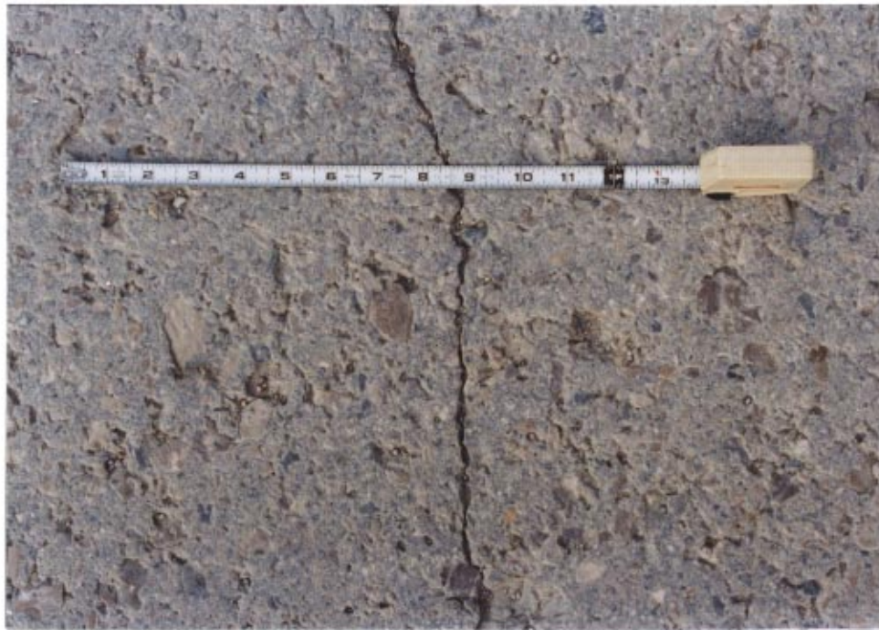
Figure 5 A typical shrinkage crack. GM Saturn plant, Spring Hill TN. Built in 1988.
