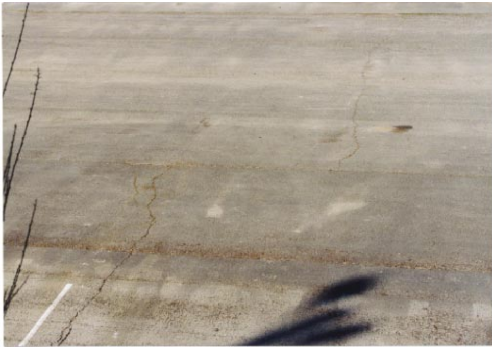
Figure 28 Typical shrinkage cracking pattern at Fort Lewis, WA.
