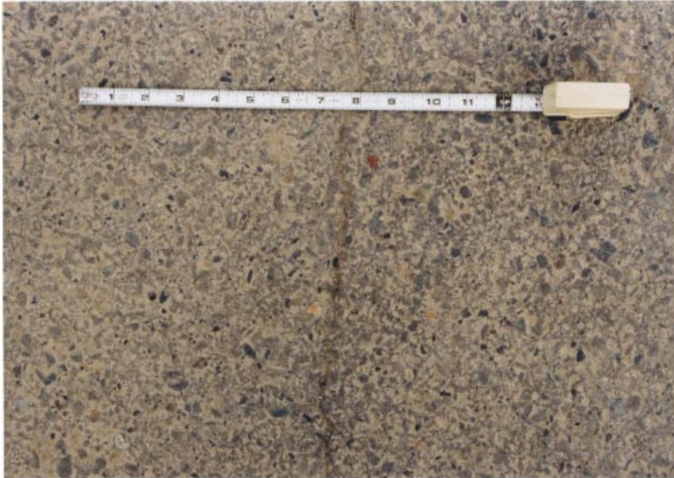
Figure 50 Shrinkage cracks in the RCC base reflect through the asphalt overlay.
