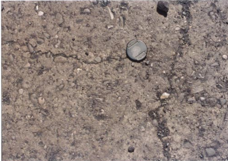
Figure 26 Shrinkage cracks become filled with coal dust.
