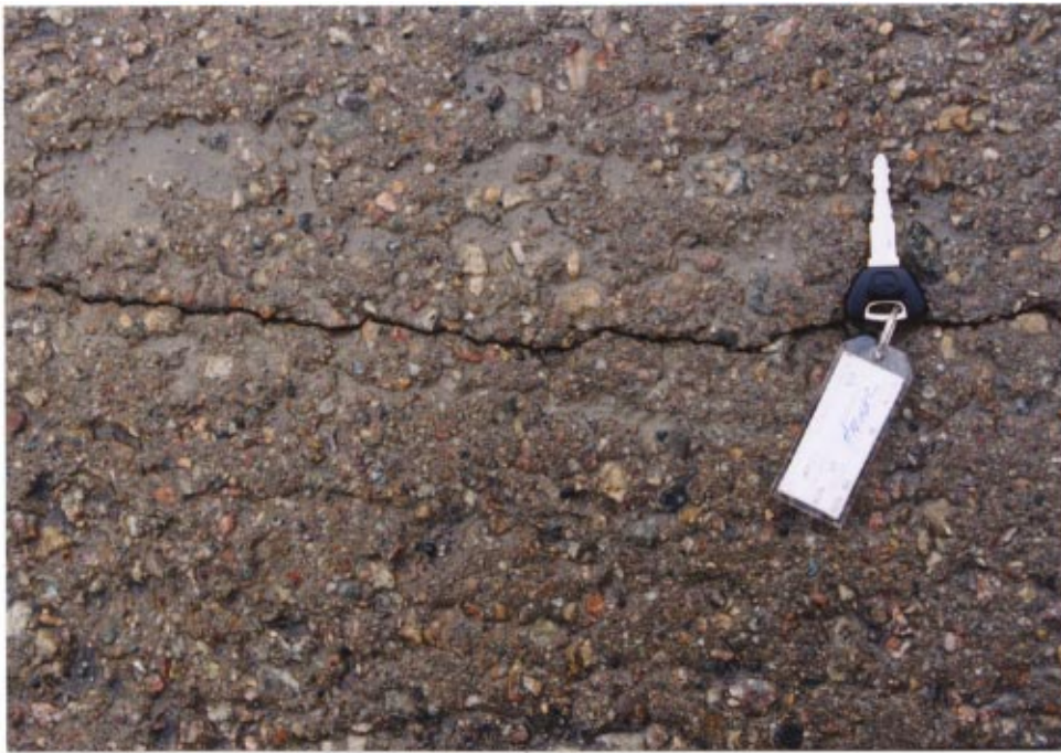
Figure 18 Typical condition of the RCC surface at Conley Terminal, Boston, MA
