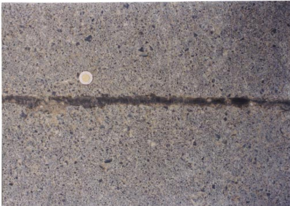
Figure 30 Bituminous joint sealant at a shrinkage crack.
