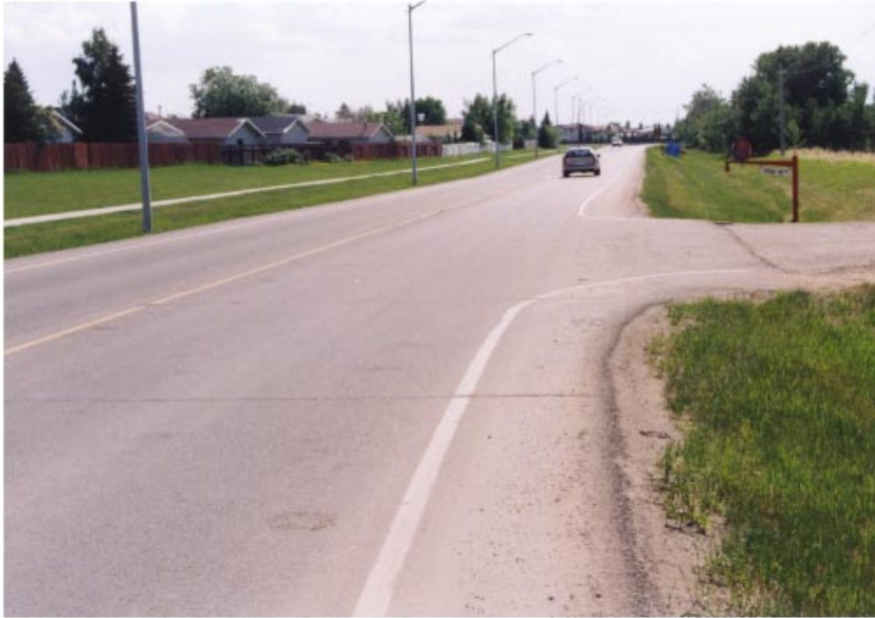
Figure 45 This experimental RCC pavement was left exposed to traffic for 3 years prior to application of the planned asphalt overlay.
