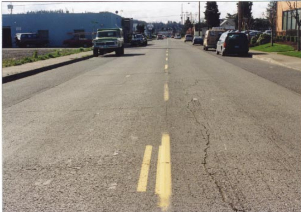
Figure 12 Collector class road, 99 th Ave., Portland, OR. This exposed RCC pavement was built in 1986. The parking lanes on each side are asphalt pavement.
