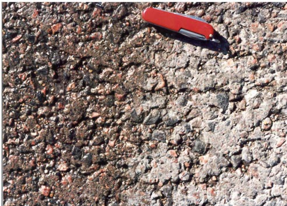
Figure 3 Surface of intermodal terminal, Denver, CO. Burlington Northern Santa Fe. Built in 1985.
