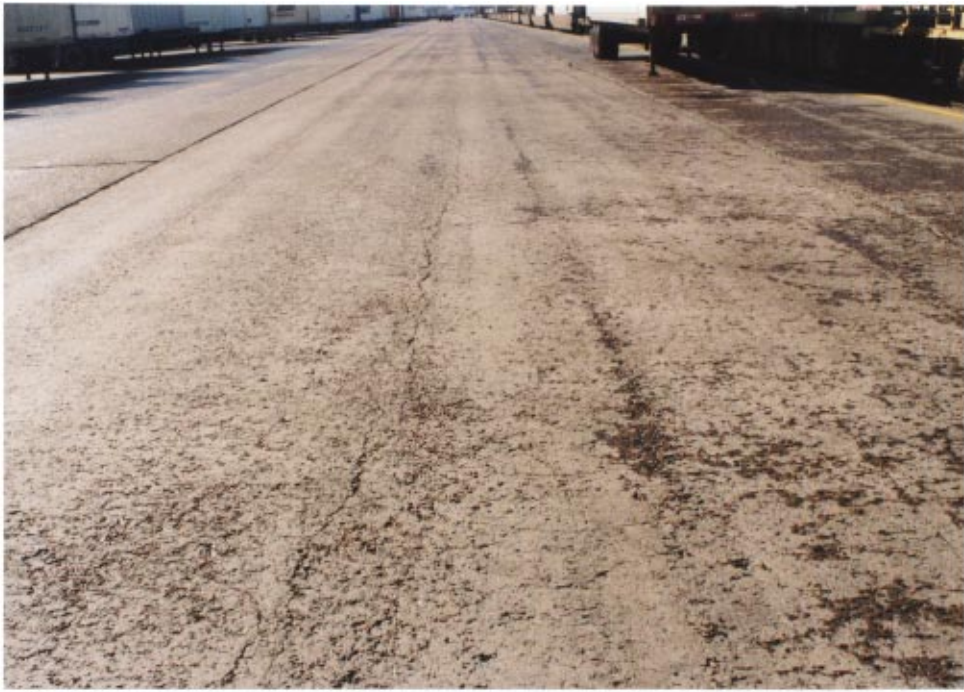
Figure 4 Variation in surface texture, intermodal terminal, Denver, CO Burlington Northern Santa Fe. Built in 1985. ( Dark areas are surface moisture )
