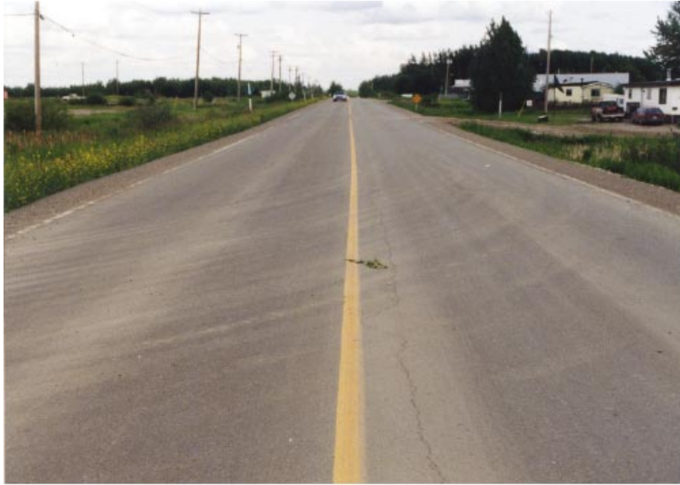
Figure 49 The street reconstruction program in the city uses RCC with an asphalt overlay.
