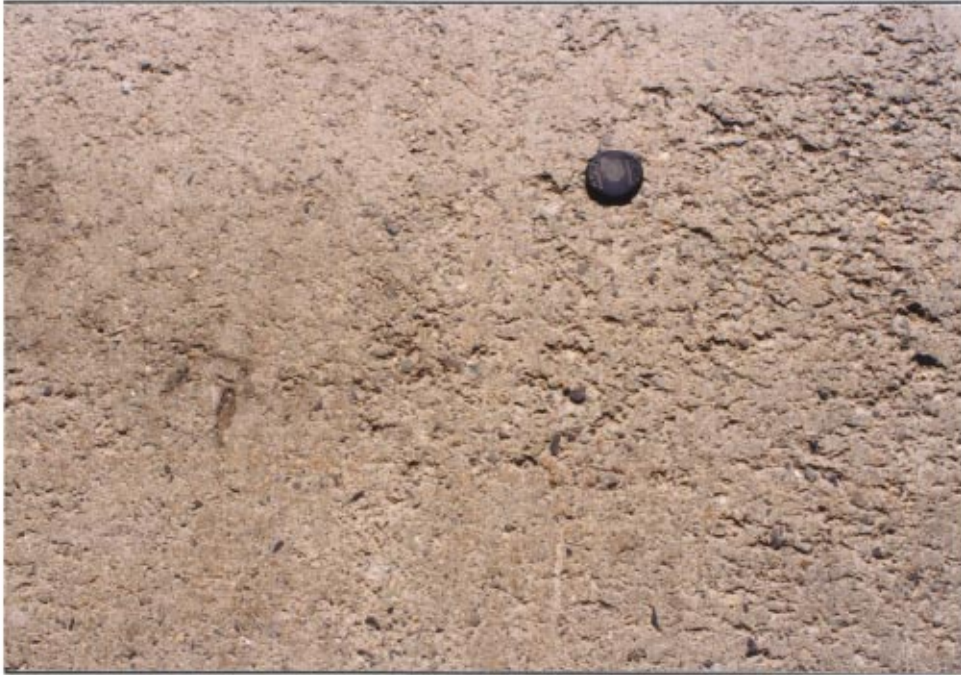
Figure 22 Operating surface of the warehouse floor, Lynnterm, North Vancouver, B.C. Built in 1989.
