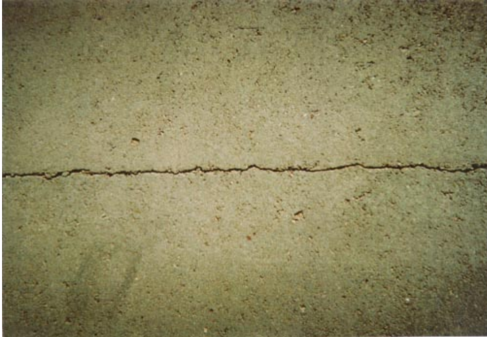
Figure 48 Bighorn Ave. at four years. The surface is in good condition and shrinkage cracks are tight.
