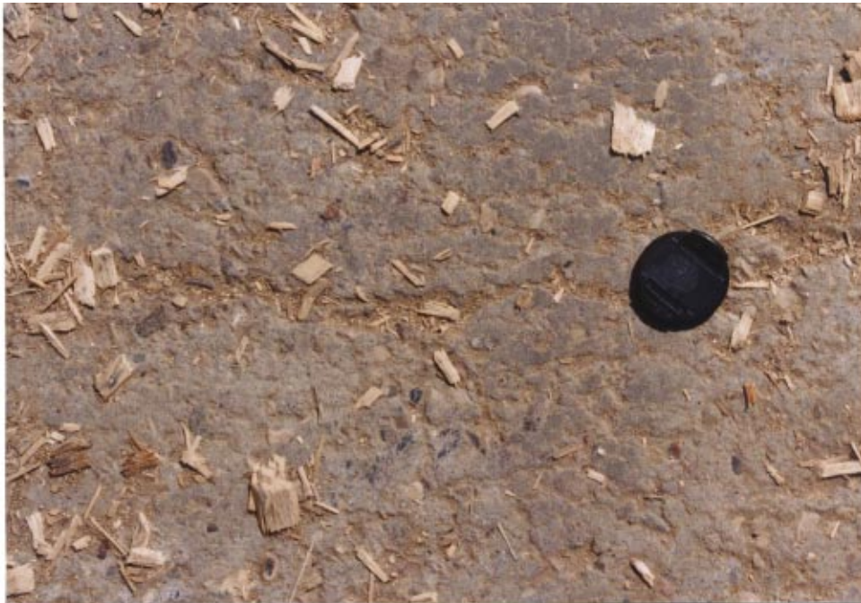
Figure 36 Wood debris fills the shrinkage cracks. The company finds no need to carry out any maintenance on the cracks.
