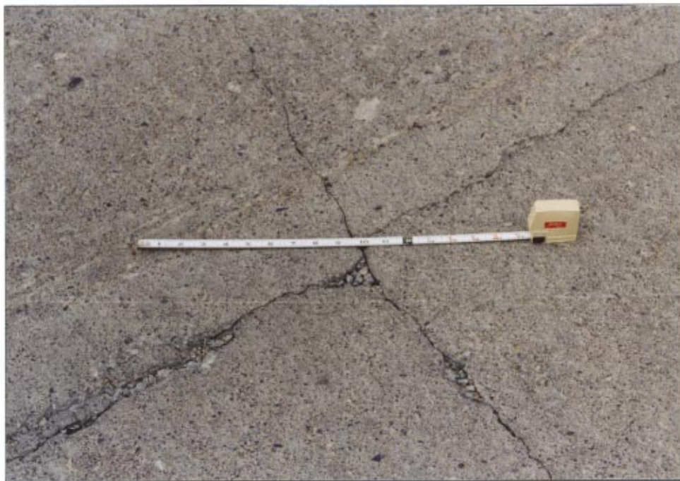
Figure 7 Chipping at the edge of shrinkage cracks from incompressible debris that enters the crack in winter. Fort Drum, NY. Built in 1988.
