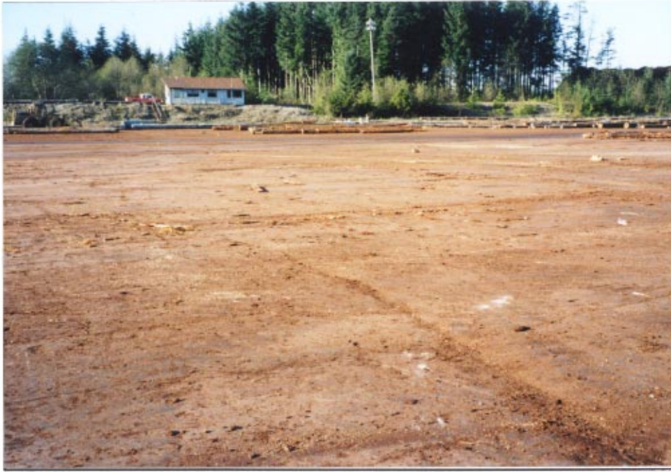
Figure 11 MacMillan Bloedel Ltd. log sorting yard, Port McNeill, Vancouver Island. No faulting at the numerous cracks in the surface. Built in 1978.
