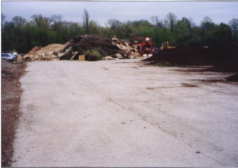
Figure 33 The heat generated in the composting process demands a pavement that will withstand high temperatures, such as RCC.
