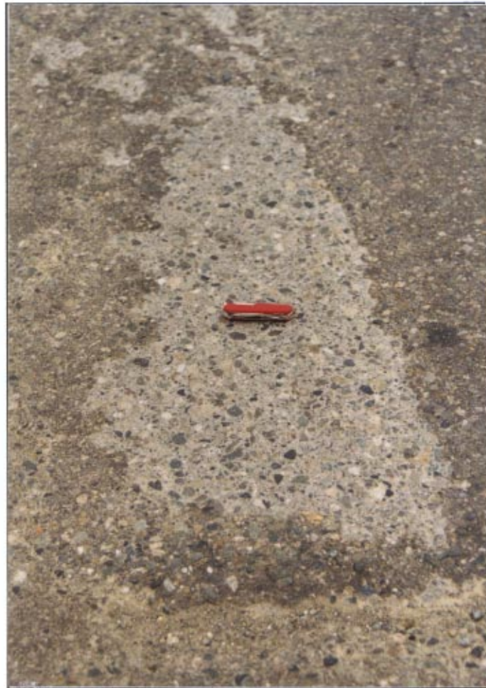
Figure 14 RCC is once again exposed on Likely Rd., Williams Lake, B.C. Built in 1987.
