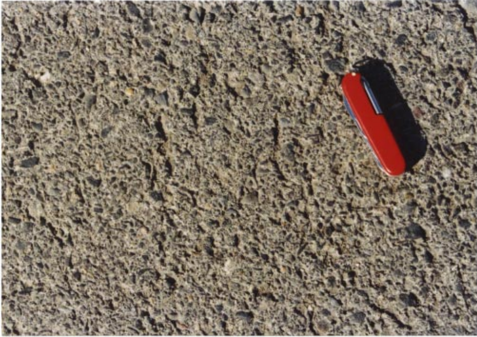
Figure 42 The surface of 99 th Ave. shows very little wear after 12 years.
