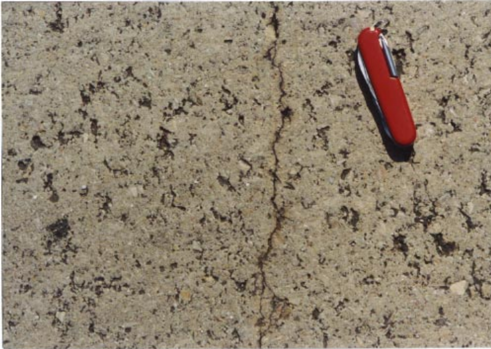
Figure 20 Shrinkage crack and surface condition, Central Freight Terminal, Austin, TX. Built in 1987.
