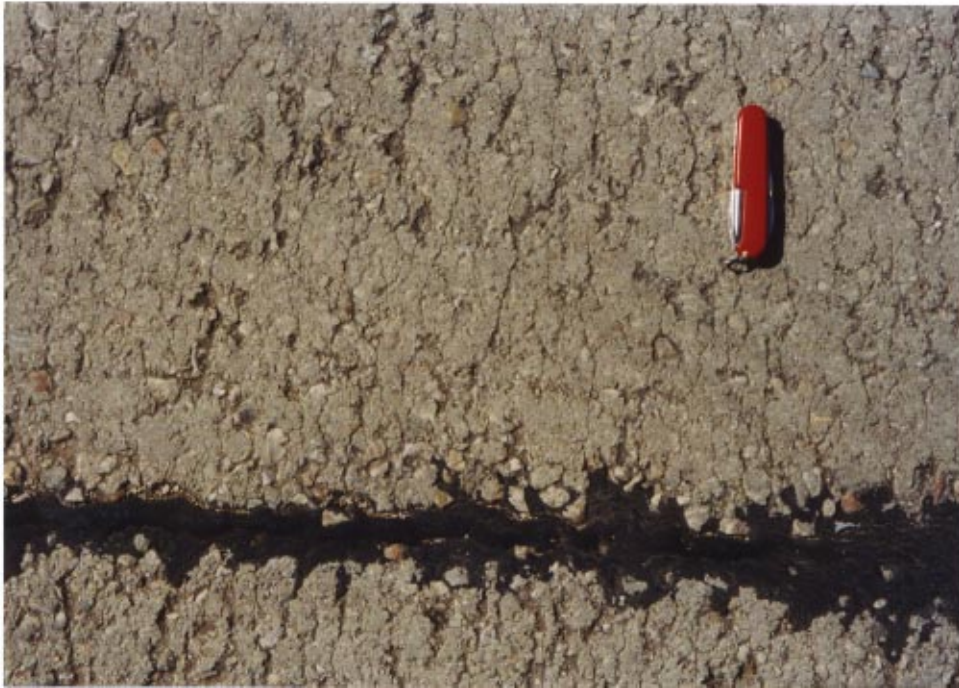
Figure 8 Joints were routed and sealed 12 months after construction was completed. Central Freight Inc., Austin, TX. Built in 1987.
