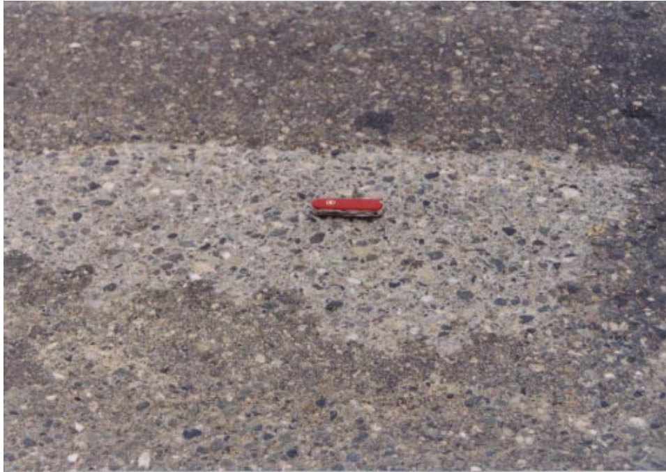
Figure 40 RCC surface is exposed again, as the 25 mm (1 in.) asphalt overlay is worn away at the intersection.
