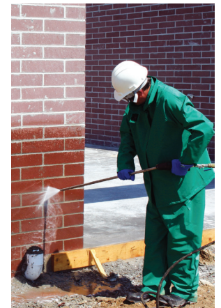
Figure 6. Pre-wetting and careful rinsing are key steps for successful cleaning with a cleaning solution. Photo courtesy of PROSOCO.
